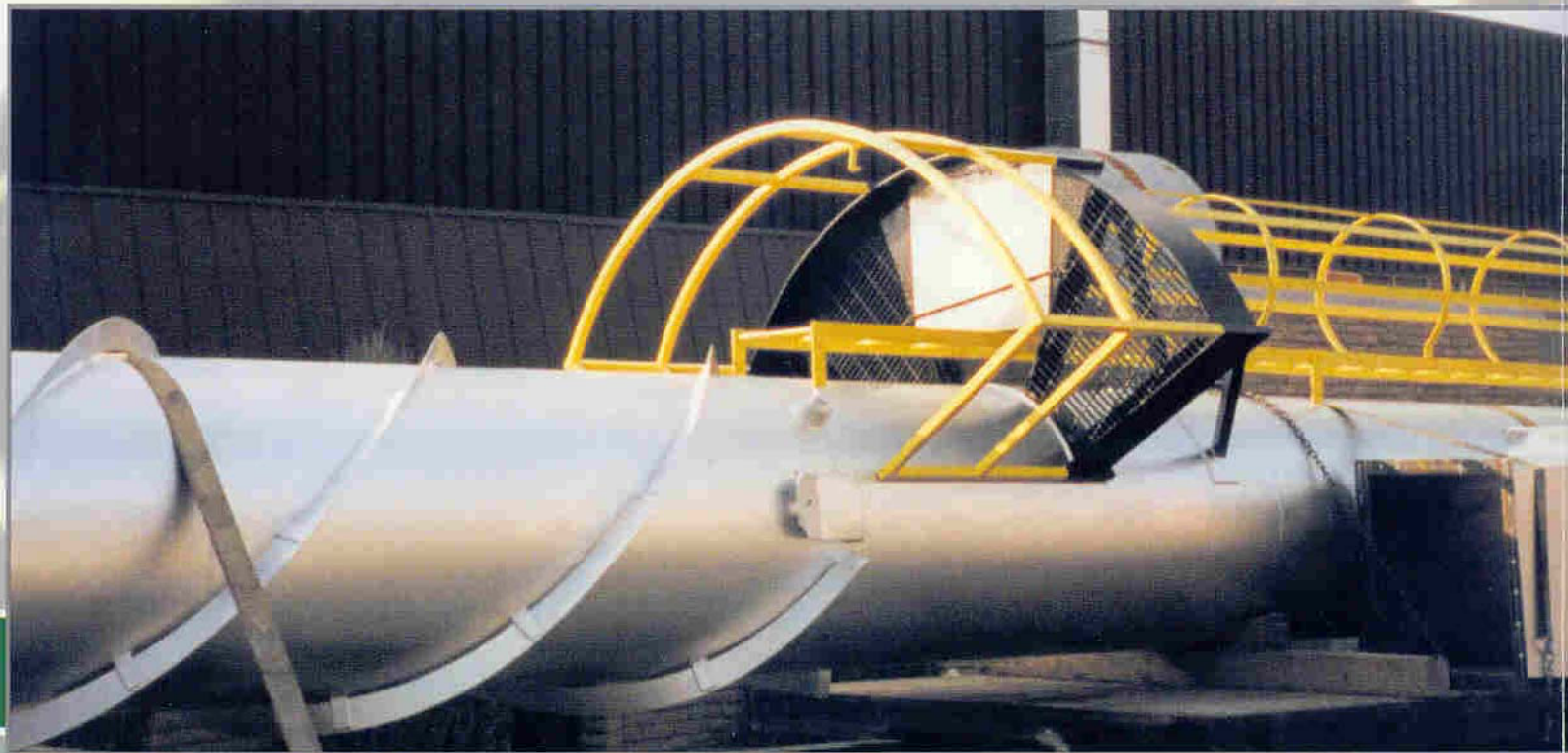
Exhaust stack for afterburner
